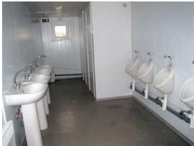
5.15-rasm. Erkaklar hojatxonasining sanitar jihozlari
